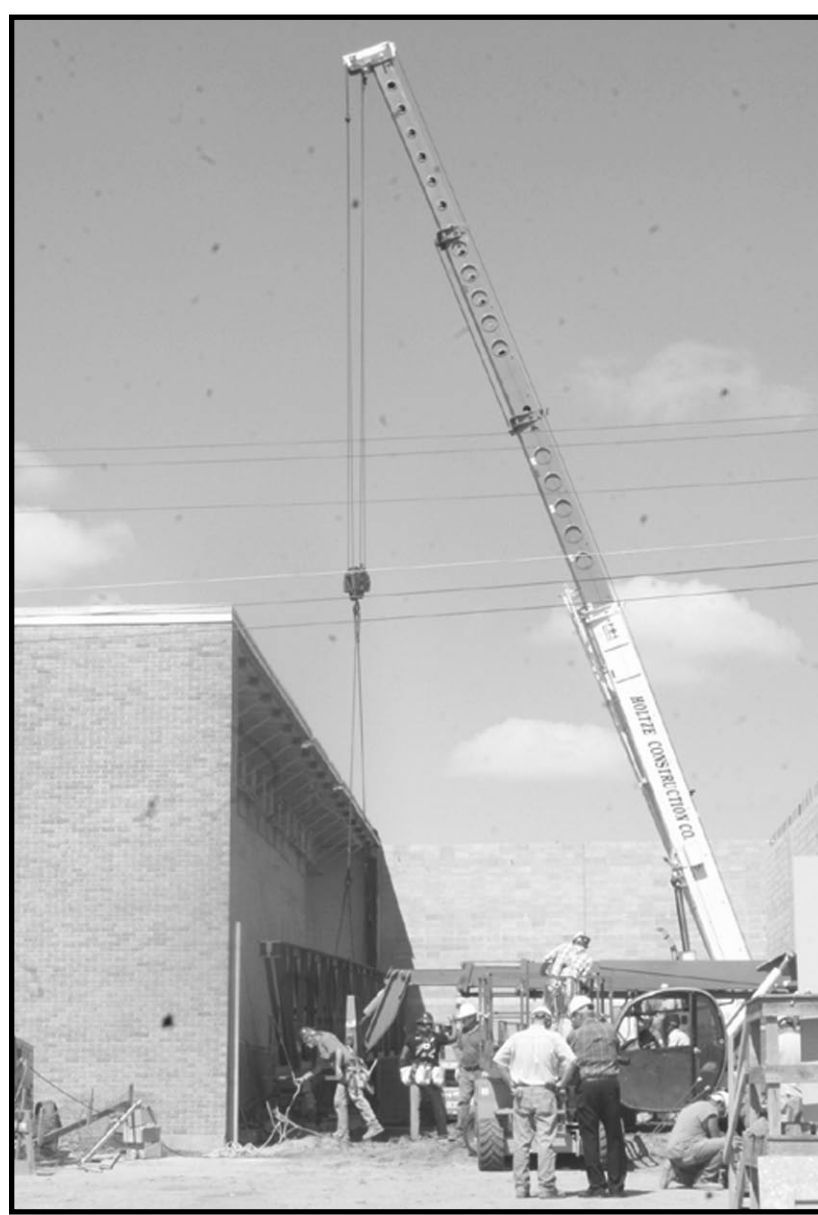
The Allen gym's new support beam was put in last week and construction crews are continuing to make progress. This week they are working on the ceiling and roof of the new addition.
